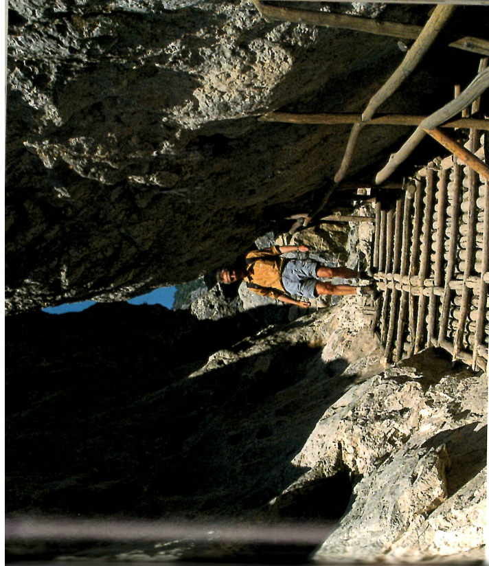
The wooden ramp through the rocky bottleneck of the gorge is not in good shape as you can see in the photo.
